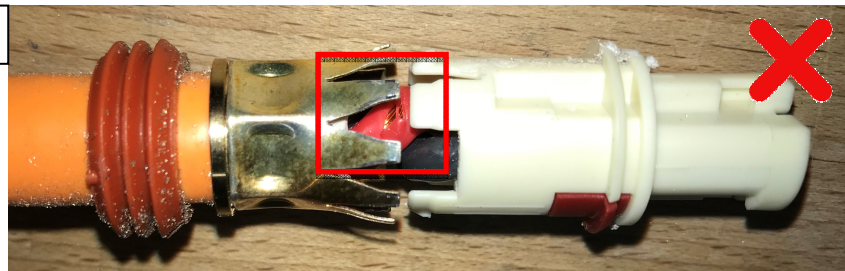
Damaged wire isolation
